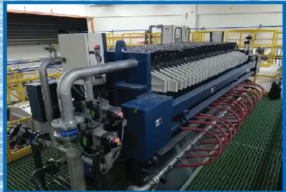
Electronic Waste Water Treatment Plant
