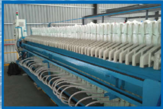
Heavy Metal Slurry WasteWater Treatment Plant
