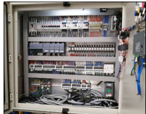
Customized Control Panel With Built In Programmable Logic Control, Frequency Inverter For Operation Of Filter Press
