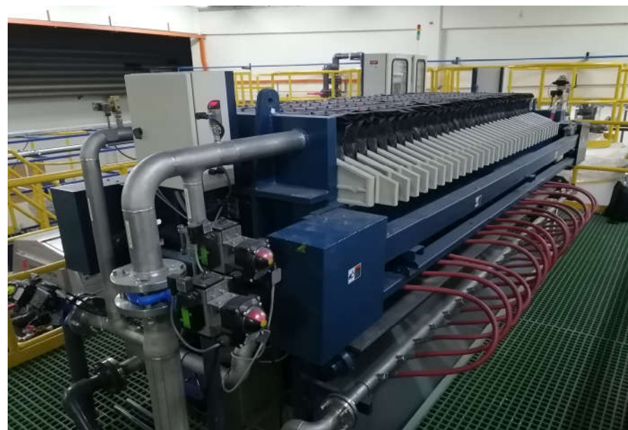
Electronic Waste Water Treatment Plant
