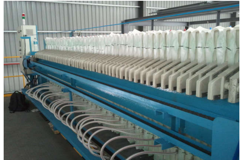
Heavy Metal Slurry Waste Water Treatment Plant
